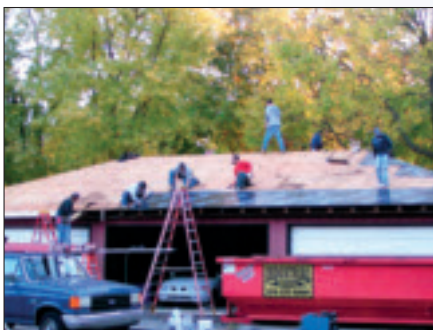
All hands on deck for the start of the Red Cross re-roof.
