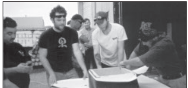
Local 58 apprentices Kyle Heikkila, Brian Cline and Adrian Sosa learn how to flash this curb correctly through hands-on training.
