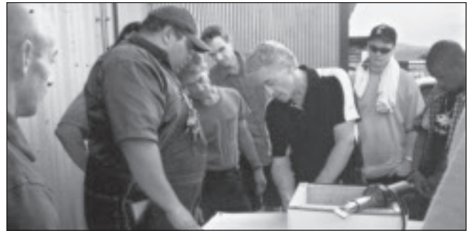
Apprentices from Local 58, Colorado Springs, CO, take note as Carlisle representative Chuck Pruitt walks through the Carlisle specifications on how to flash a curb.
