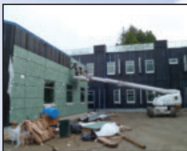
College of Marin Science Building has partial installation of Trespa panels on the left-hand side.
